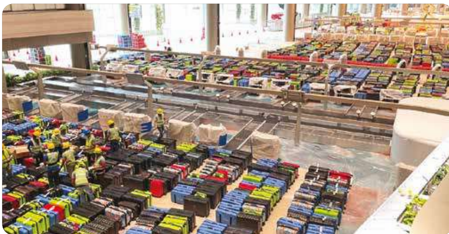
CAG conducted intensive tests of the upgraded baggage handling system at T2 before its reopening.
