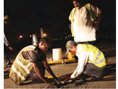
Regular airfield maintenance ensures the safe use of the airfield infrastructure as aircraft traffic increases at Changi Airport.
