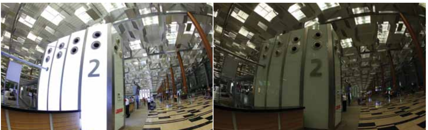
Lights at Terminal 3's Departure Hall and Departure/ Transit Mall were dimmed by 80%
