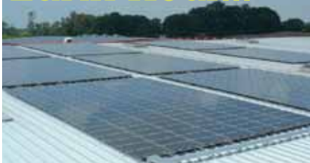
Solar photovoltaic (PV) panels installed on Budget Terminal rooftop
