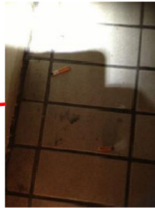
Cigarette butts found behind staircase landing
