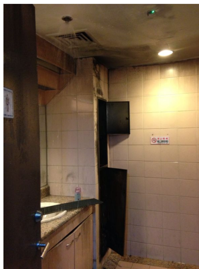
Figure 2 – Heated Smoke from the dustbin fire activated the fire sprinkler and resulted in smoke damage to the property
