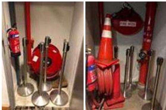
Illegal storage in hose reel cabinets
