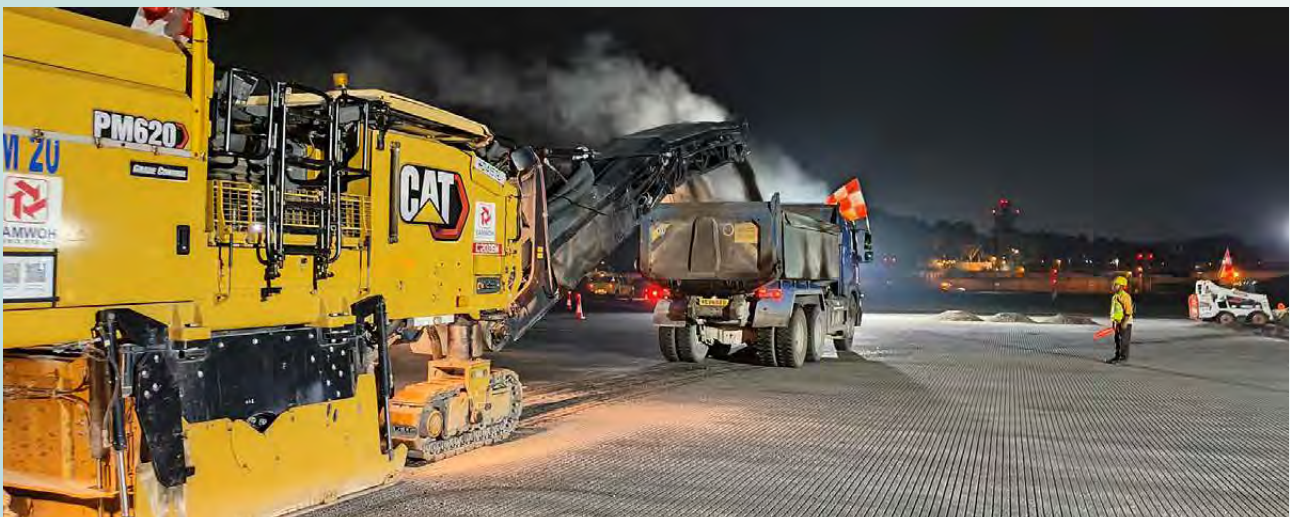
CAG started resurfacing works for Runway 1 to ensure operational safety and reliability.
